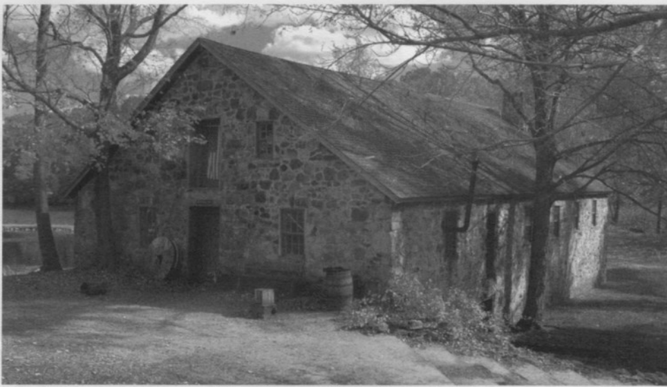
Waterloo's historic stone gristmill has been the focus of state-funded masonry repairs and repointing during the course of this summer
