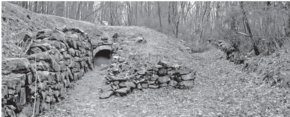
This 2007 photo of the tailrace tunnel and bypass channel at Plane 2 East was taken before the Phase I restoration stabilized the turbine chamber. Since then, these stone walls have continued to deteriorate and the whole area has overgrown by invasive vegetation. The newly funded Phase II restoration work will fix these problems and make the site more accessible for visitors.
