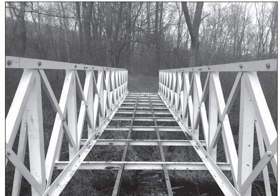
BELOW: The bridge framework is now in place awaiting the installation of its wooden floor boards.
