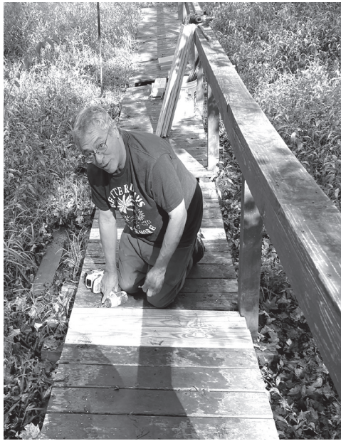
ABOVE: WCPF volunteer Steve Deldonno works to repair the boardwalk needed to complete this section of Greenway trail.
