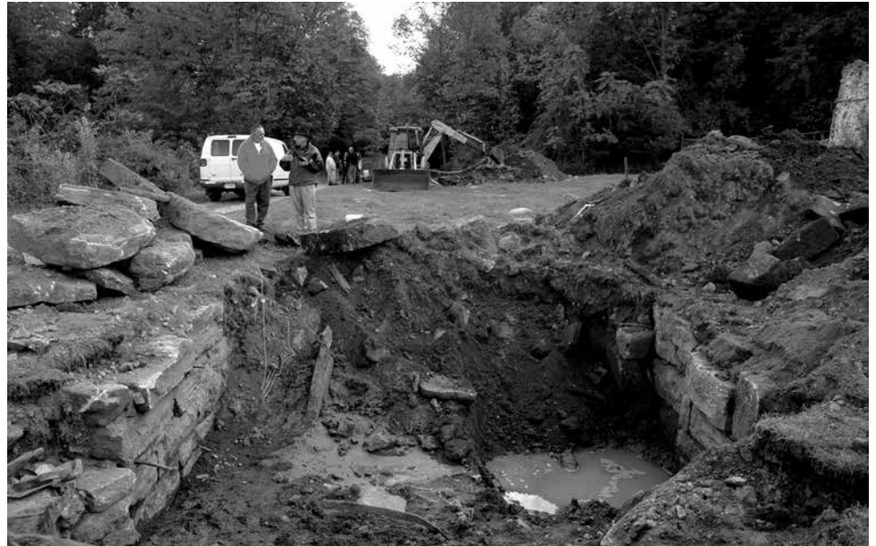
In 2006 project manager John Manna and local historian Richard Cramond visit the lock site to inspect the work as a team of archeologists use a backhoe to partially clean soil from the upper and lower ends of the lock chamber. To everyone's surprise, they discovered that the lock had been only partially dismantled and that the lower walls and substructure were in good condition.
