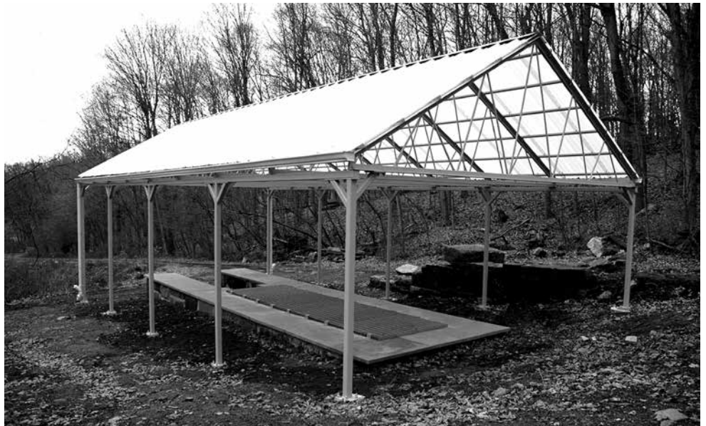
To complete the project, this pavilion was erected over the top of the turbine shaft to prevent ground water from once again working its way into the stonework below.
