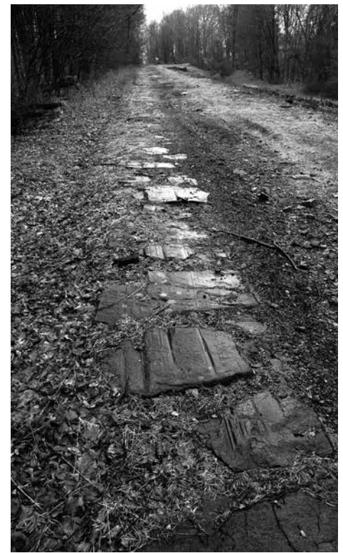
This line of sleeper stones, scarred from years of use, stretch the full length of the slope of Plane 2 East.
