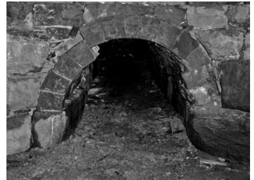
In the photo above, the stones in the tailrace arch without a proper footing have slipped out of alignment and the arch was about to fail.
