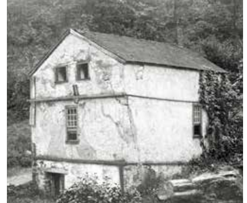
By the early 1900s, the tender's house at Lock 2 East was in poor condition. To prevent the building from collapsing, the canal company used pieces of inclined plane rail and lengths of cable to hold the building together. The plans to rebuild the house included reproducing the stabilization system.
